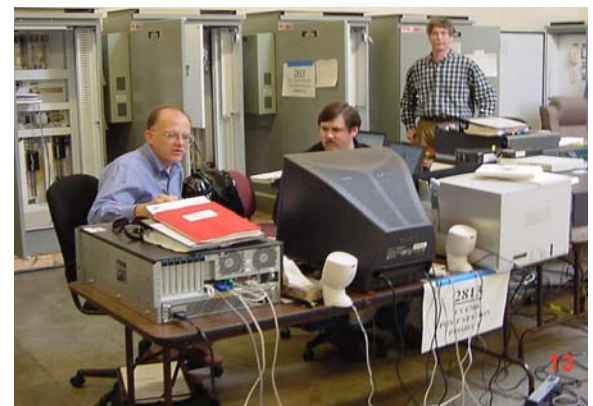
Central Contra Costa County Sanitary District SCADA Factory Demonstration Test
